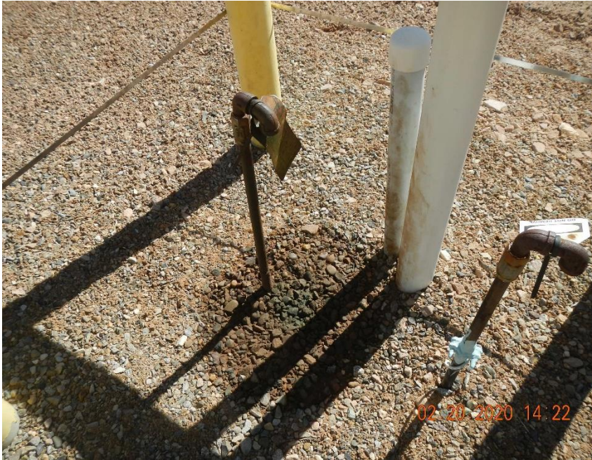
Staining below flow line vents from lubricant used during installation of internal sleeve.
