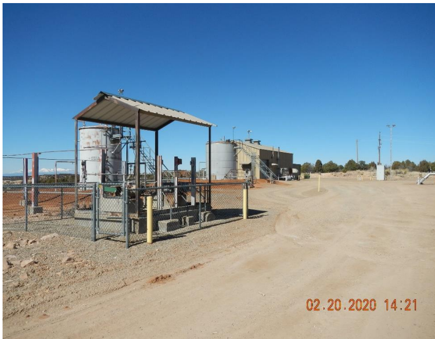
YB Cluster CDP and tank battery.
