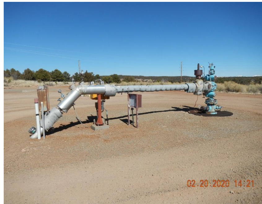
YB-3 well head and flow line.
