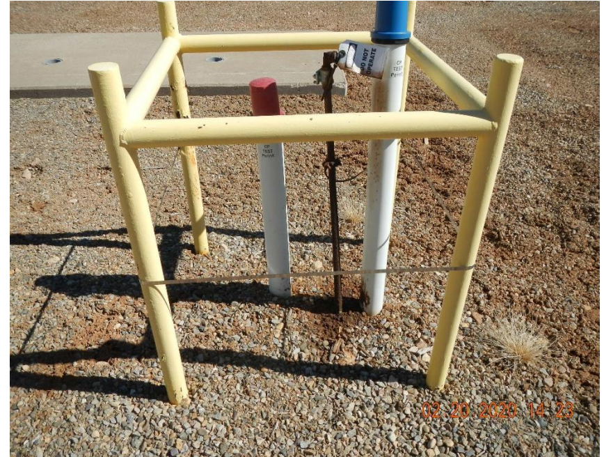
Lubricant weeping out of flow line vents.
