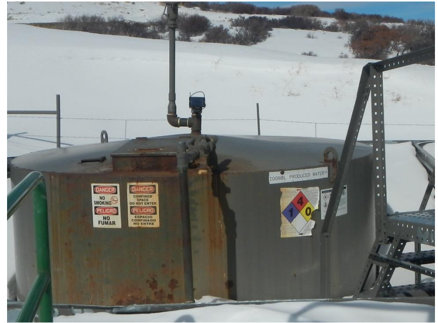
Capacity label has been replaced.
