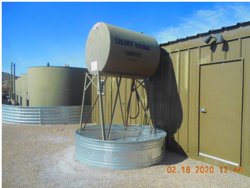
Secondary containment of chemicals at pump housing
