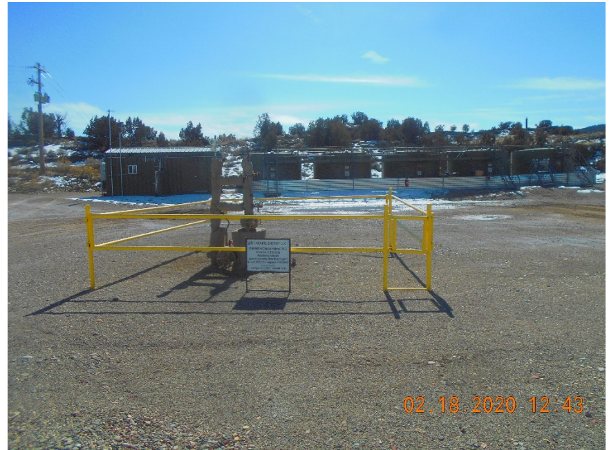
Injection wellhead with fence and sign. Pump housing and tank battery in background.
