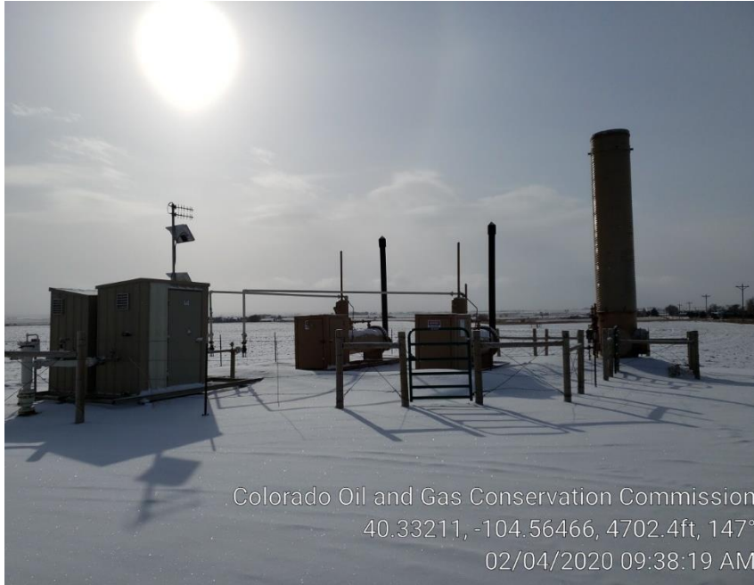
Photo #3 Separators, ECD, & Meter Runs
