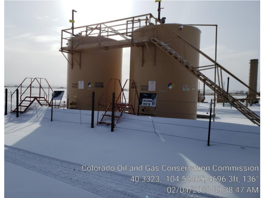
Photo #4 Tank Battery
