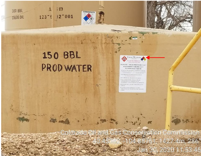
Photo 3: NFPA placard installed
