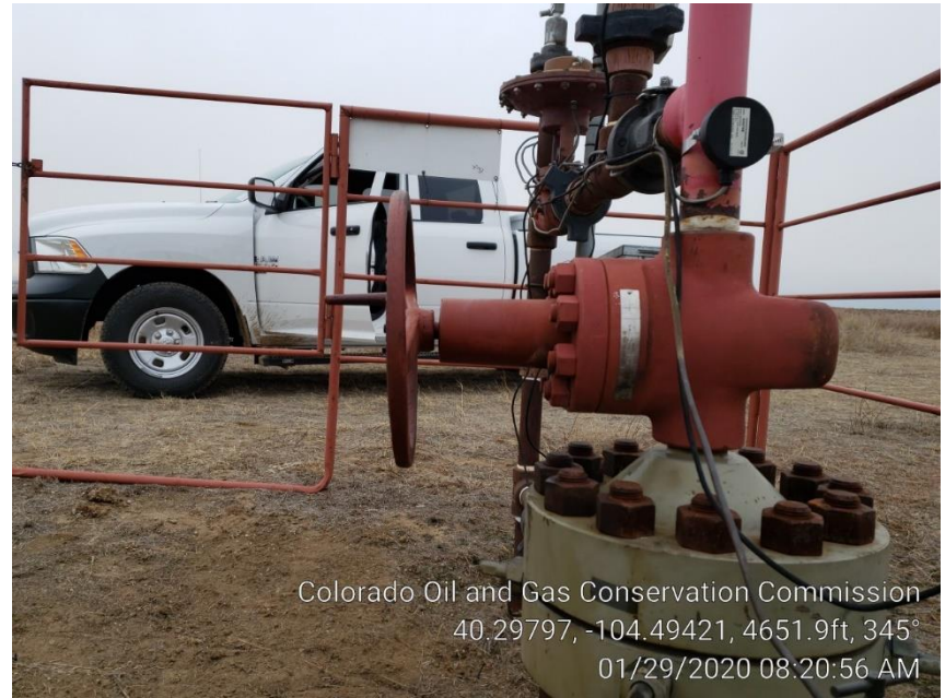
Photo #2 No leaking Master Valve
