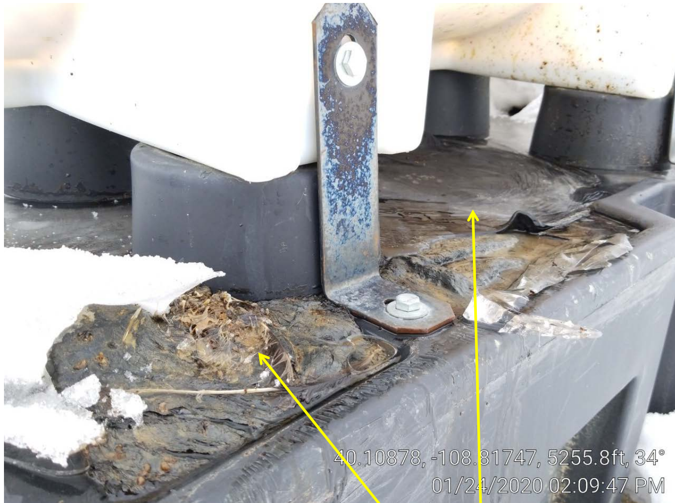
Photo 3. Container secondary containment with dead bird & tar like substance
