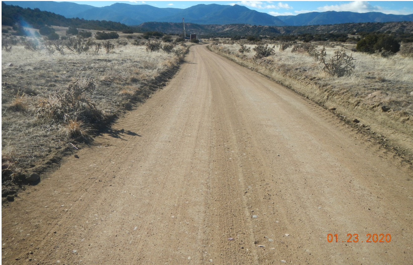
Photo 1. Facing west along the access road. The road has been repaired and road base has been spread along the road and is now compacted and stabilized.
