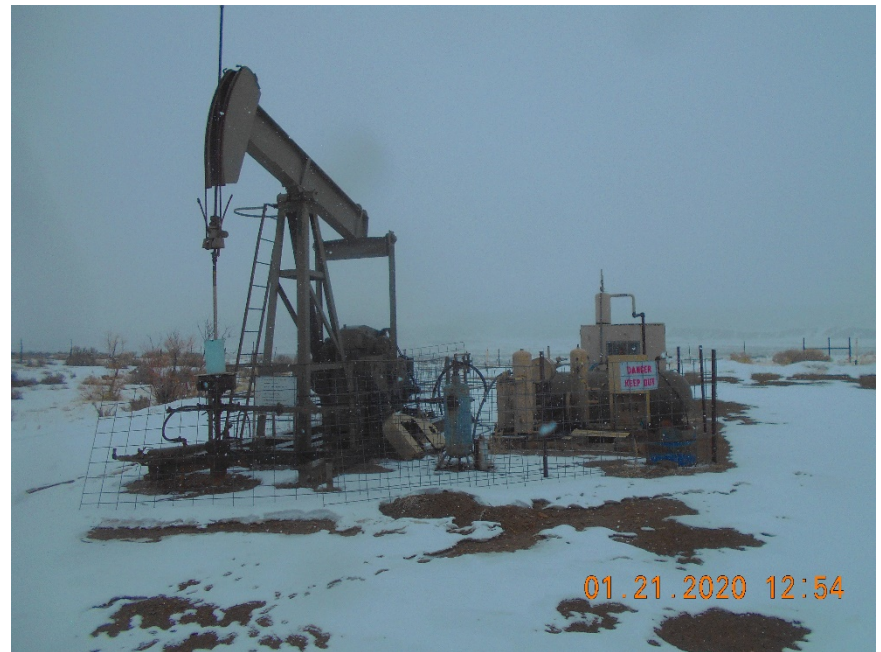
Pump jack with sign
