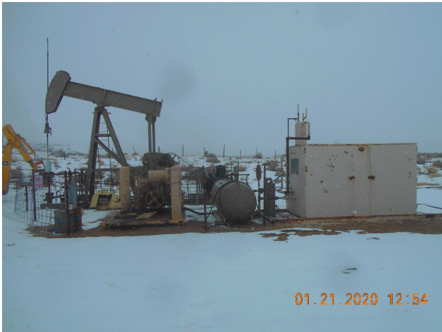
Compressor and Separator
