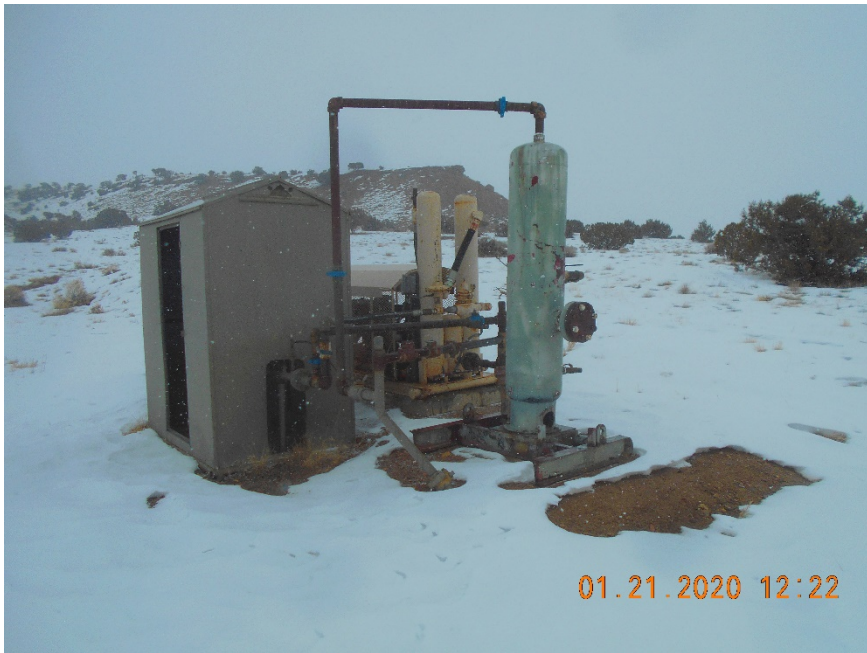
Meter housing and Compressor
