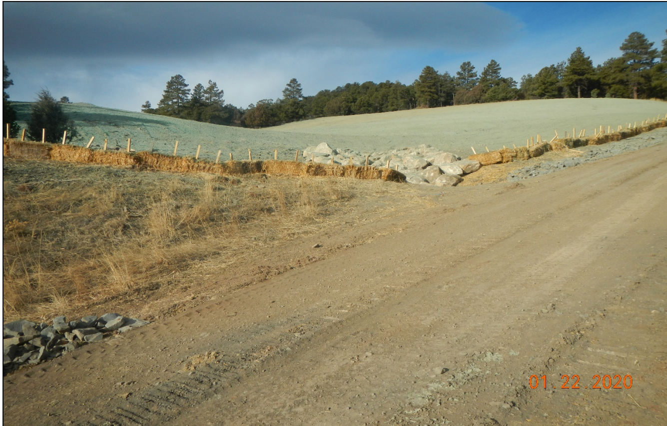
Photo 5. Facing northwest toward the location which has been recontoured and reclaimed. The location has been hydromulched and stormwater controls are installed around the perimeter and drainage areas.
