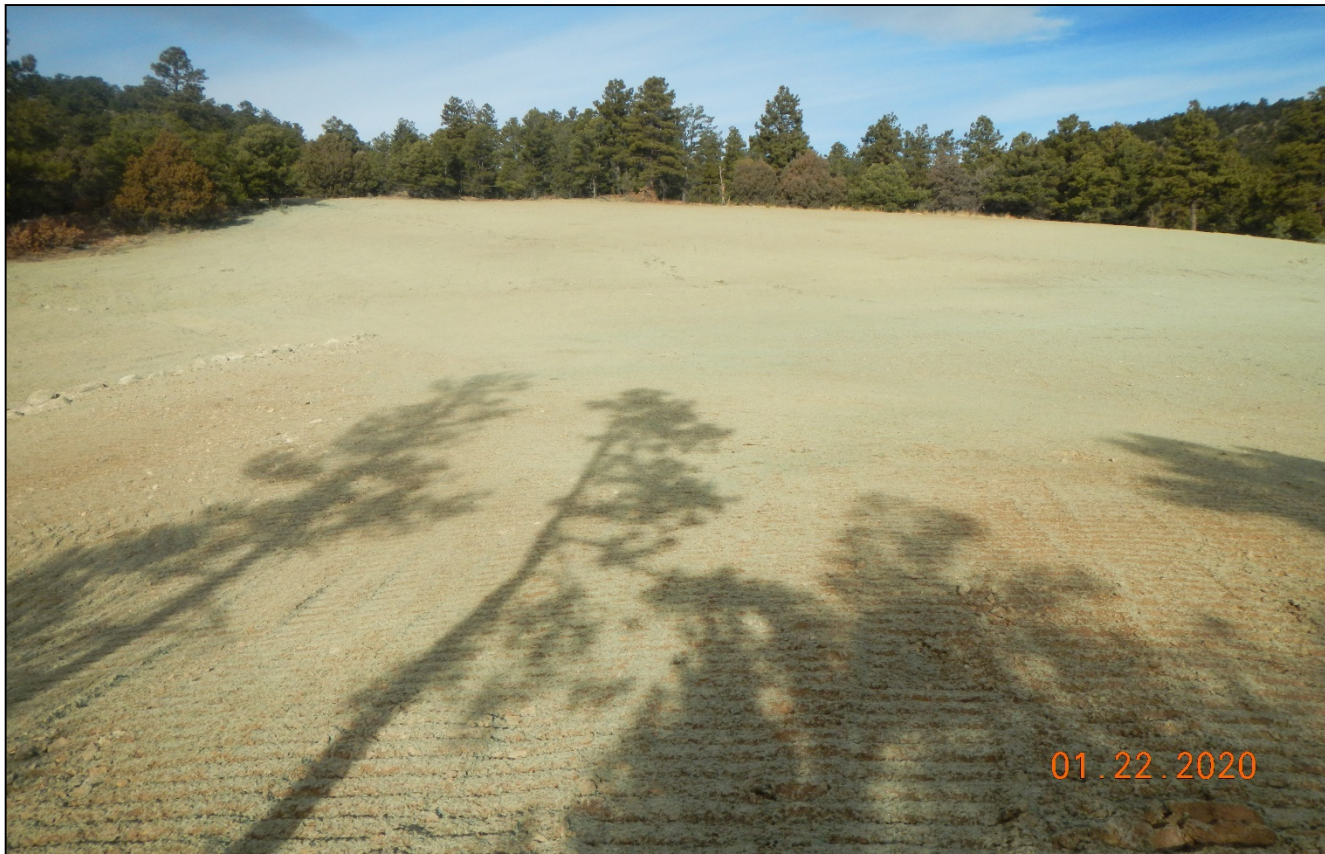
Photo 10. Standing at the bottom of the location facing north. The soils were properly tracked and hydromulched.
