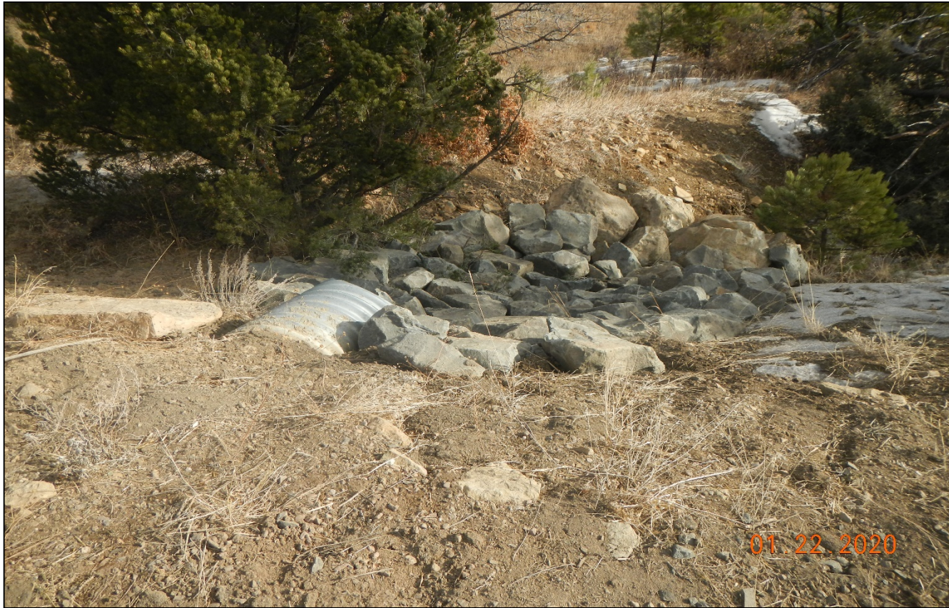
Photo 4. The culvert outlet has been cut closer to the surface and rock rip/rap outlet protection has been installed.
