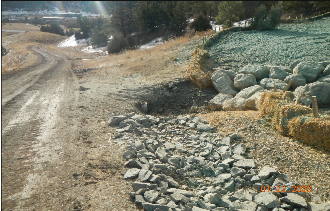
Photo 8. Facing southeast near the bottom of the location. Stormwater controls are installed along the side of the road and perimeter of the location Stormwater is directed toward the culvert at this point.
