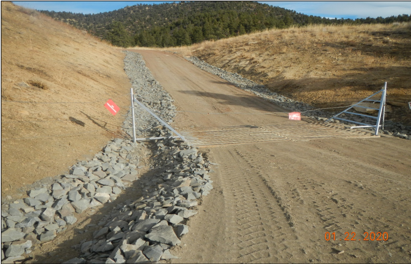
Photo 1. Facing north at the beginning of the access road. Additional rock rip/rap has been installed along the side of the road to prevent erosion.
