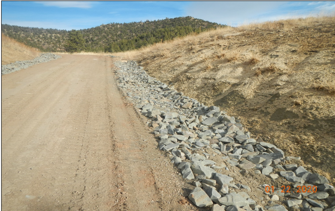
Photo 2. Facing toward the side of the access road as it ascends up the steep grade. Rock rip/rap and check dams have been installed along the road. The sides of the slope have been seeded and hydro mulched.
