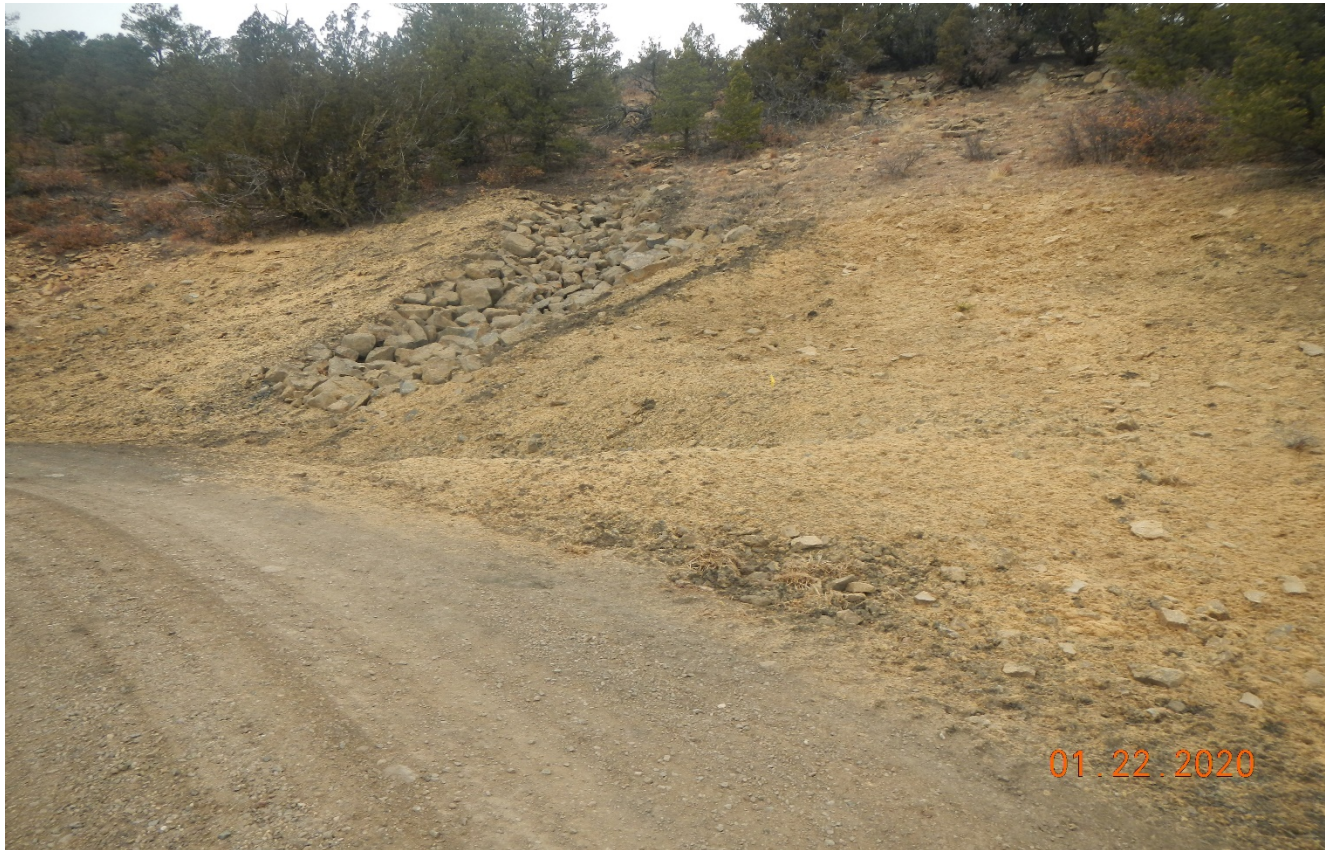
Photo 2. The area of erosion identified along the access road has been repaired. Rock rip/rap was installed and the cut slope is seeded and hydromulched.
