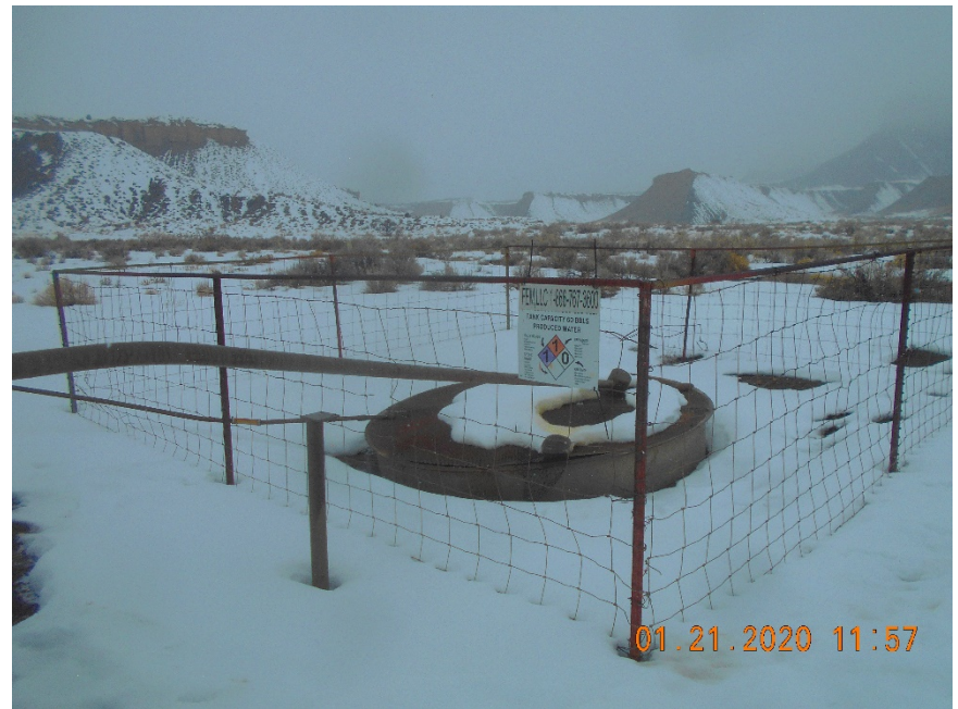
Blowdown tank with fence and sign
