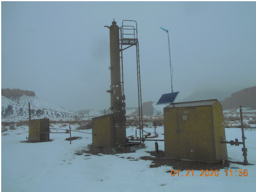
Separator, Dehydrator with blowdown tank, Meter housing
