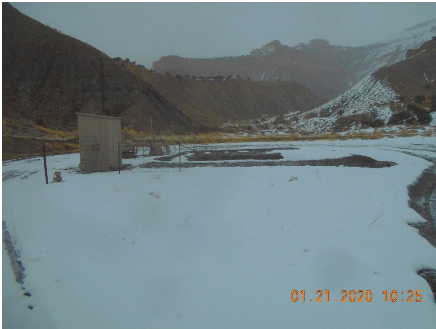
Location overview looking NE. Meter housing with sign, Separator, Produce water tank and pit.
