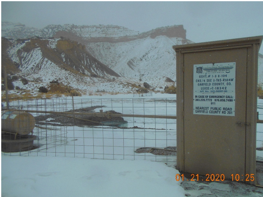
Meter housing with sign
