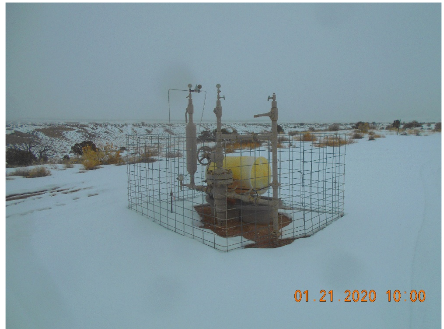
Wellhead with fencing
