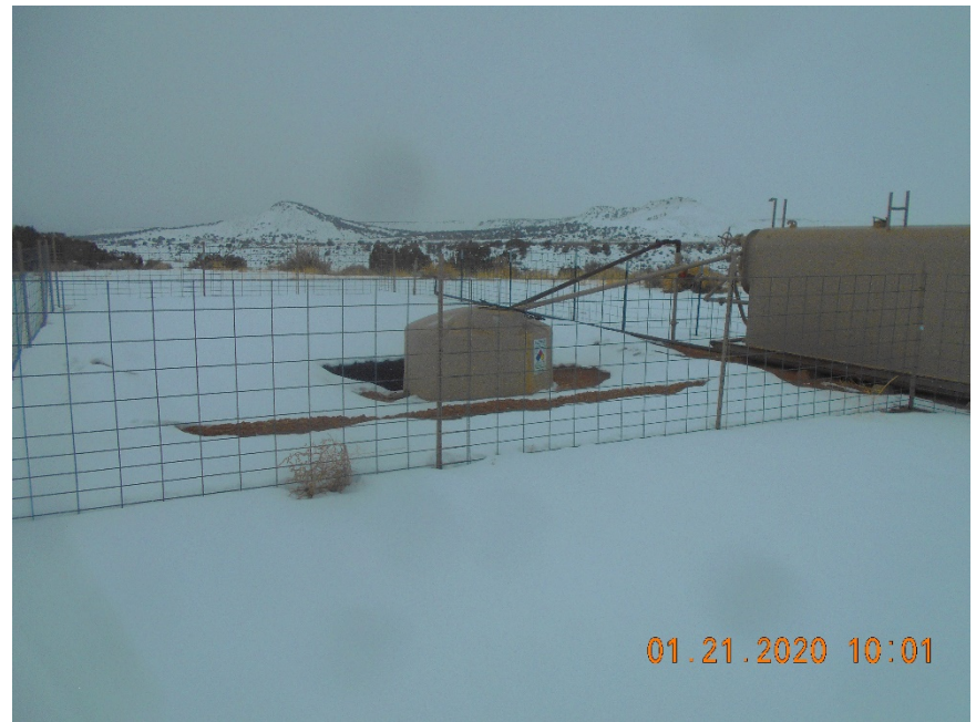
Produced water tank and blowdown pit
