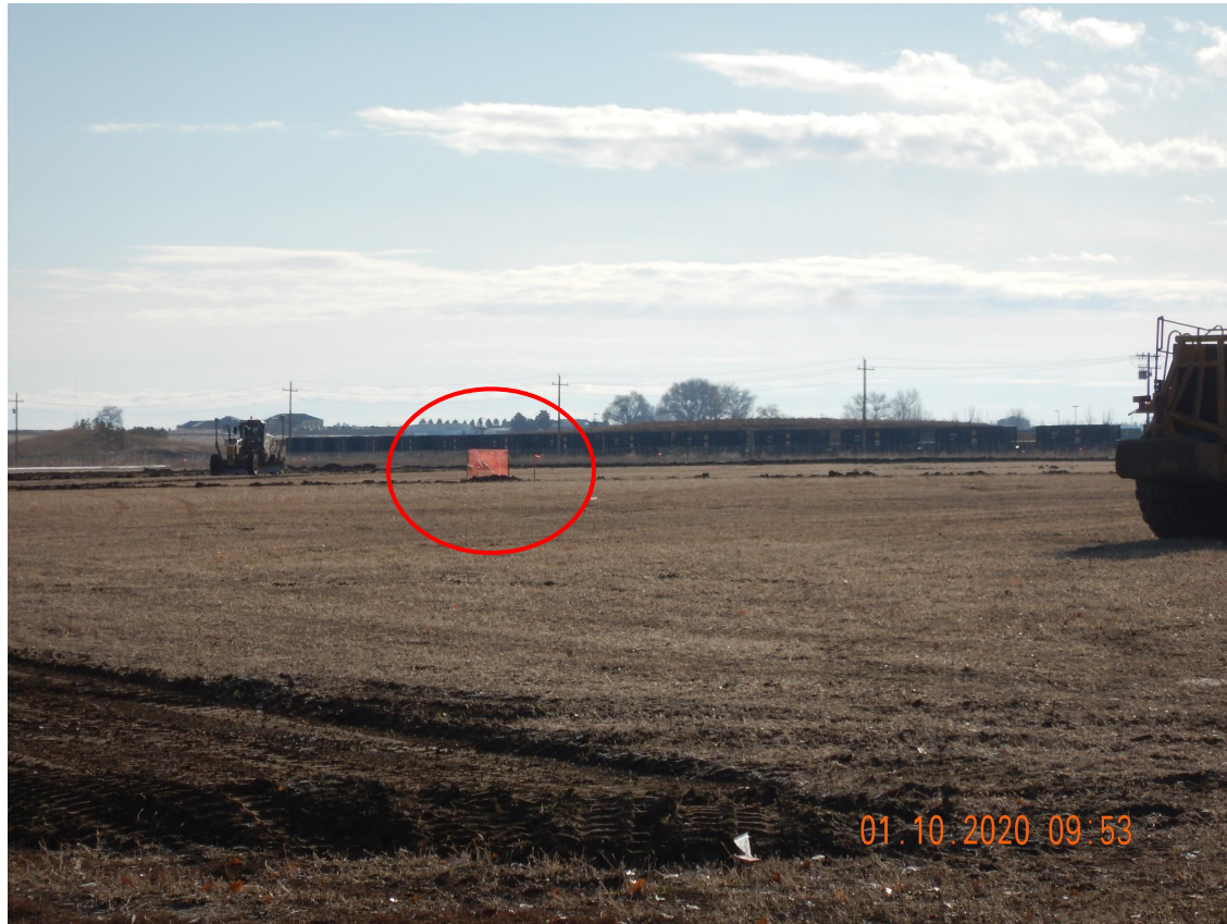
Photo 3. Photo taken from the northwestern perimeter of the new location (Location ID 470396) on 1/10/2020, facing East. Photo illustrates construction activities underway in relation to the re-plugged well circled in red.
