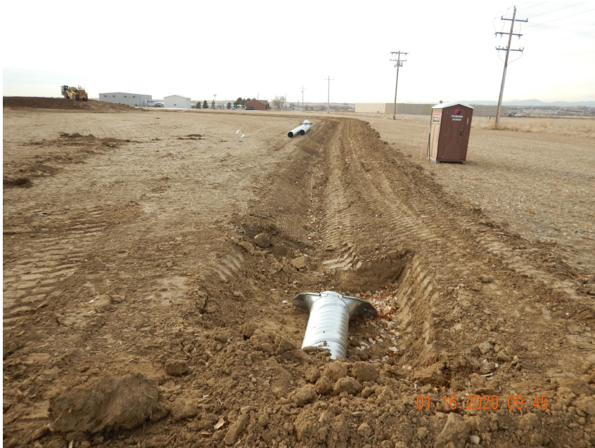
Photo 10. Photo taken from the Northwestern perimeter of location on January 16, 2020, facing South. See comments under Photo 9 regarding the ditch and berm BMP. Operator still in-process of installing inlet/outlet protection for the above culvert.
