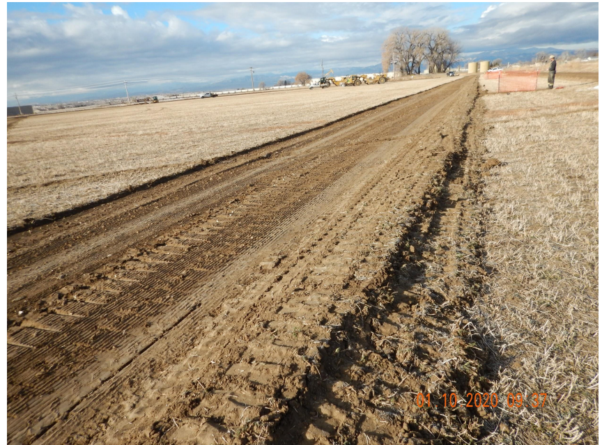
Photo 6. Photo taken from the Northeastern perimeter of location on January 10, 2020, facing West; towards Larimer County Road 1. See comments under Photo 1 regarding the ditch and berm BMP.
