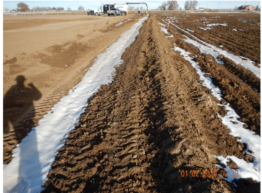
Photo 4. Photo taken from the eastern perimeter of location on January 10, 2020, facing Northwest. See comments under Photo 1 regarding the ditch and berm BMP.
