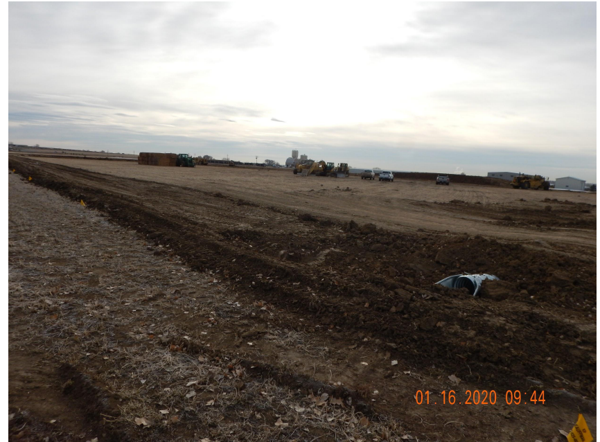
Photo 9. Photo taken from the Northwestern perimeter of location on January 16, 2020, facing Southeast. Operator has completed the installation of the ditch and berm BMP. Operator has stabilized the berm portion of the BMP with equipment tracking.
