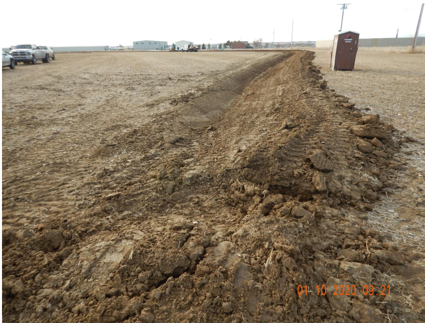
Photo 1. Photo taken from the Northern perimeter of the location on January 10, 2020, facing South. Photo illustrates the beginning of a ditch and berm BMP; however, Operator had not yet completed installing the BMP at the time of this inspection.
