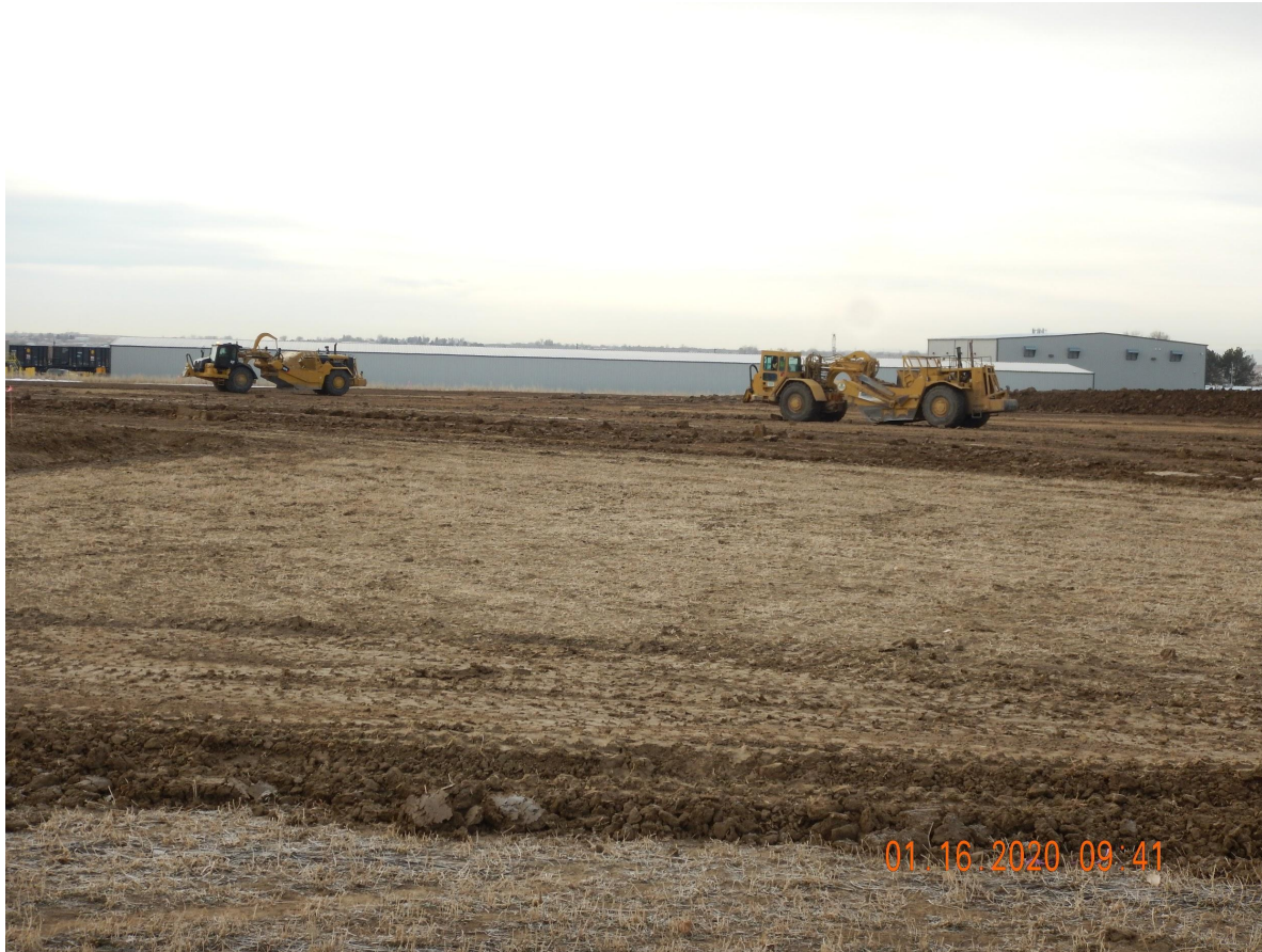
Photo 7. Photo taken from the Northern perimeter of location on January 16, 2020, facing South. Photo illustrates Operator conducting topsoil salvage operations along the eastern portion of location.
