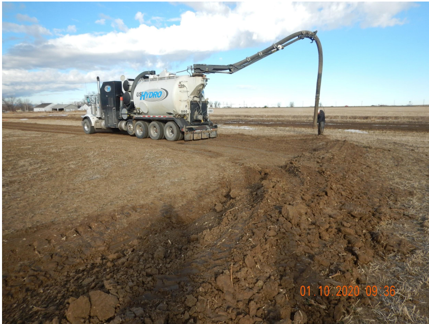
Photo 5. Photo taken from the Northeastern perimeter of location on January 10, 2020, facing North. Photo illustrates a hydro excavation operation. Operator is trying to delineate where an irrigation tile drainage is located so damage does not occur when installing the sound walls.
