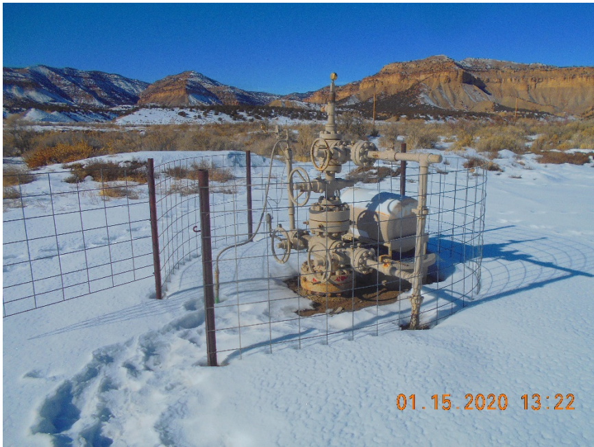
Wellhead with fencing
