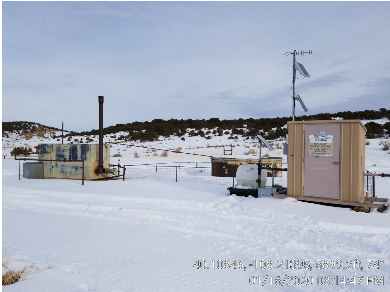
Photo 3. Meter building, blowdown tank, and separator.
