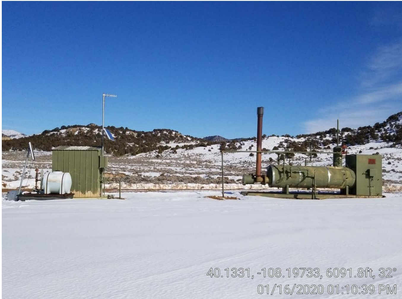
Photo 3. Separator & meter building.
