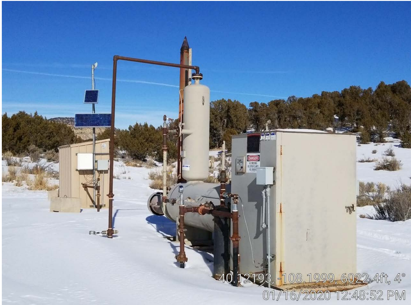
Photo 2. Separator & meter building.
