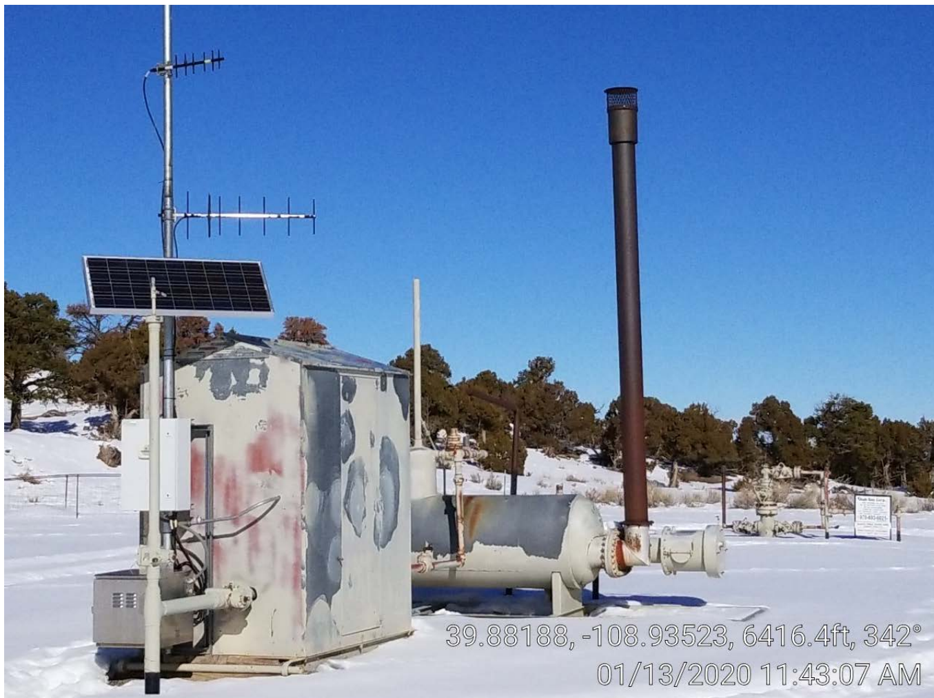
Photo 3. Separator, meter building, and well head.
