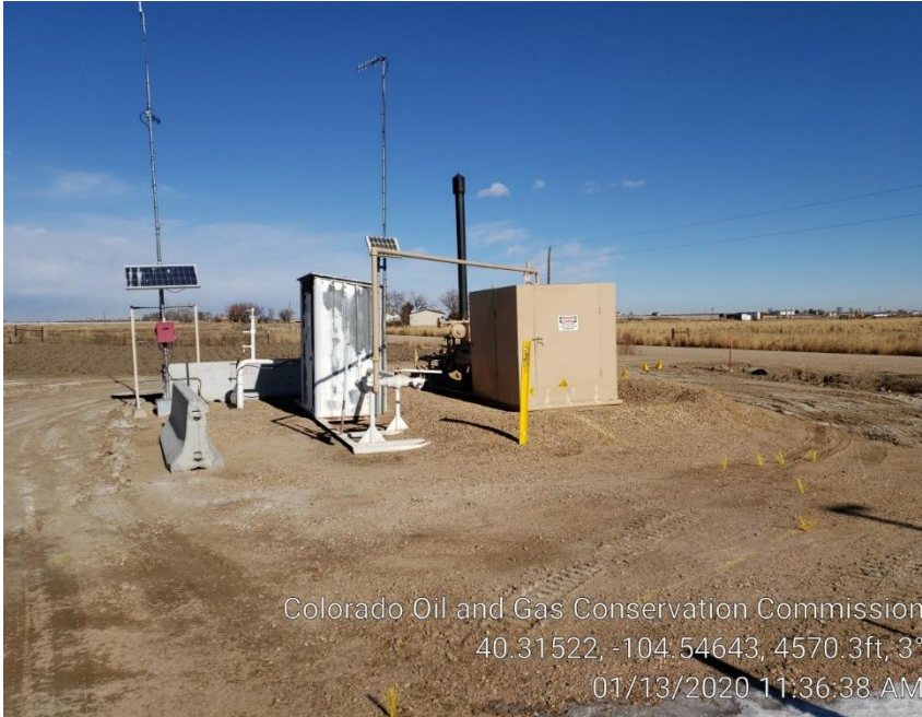
Photo #2 Separator & Meter Run
