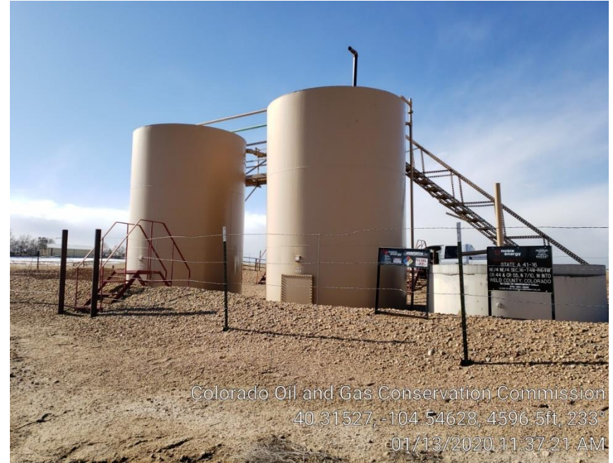
Photo #3 Tank Battery
