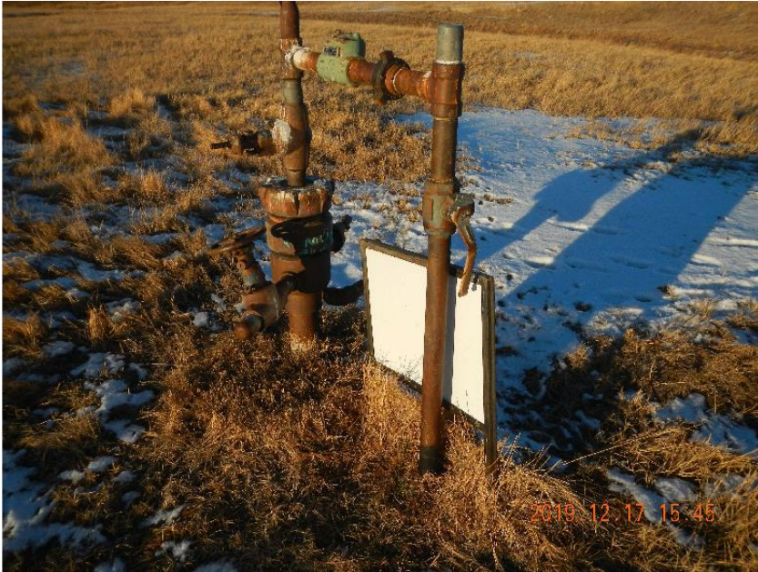
Photo 3: Backside of wellhead and tree.
