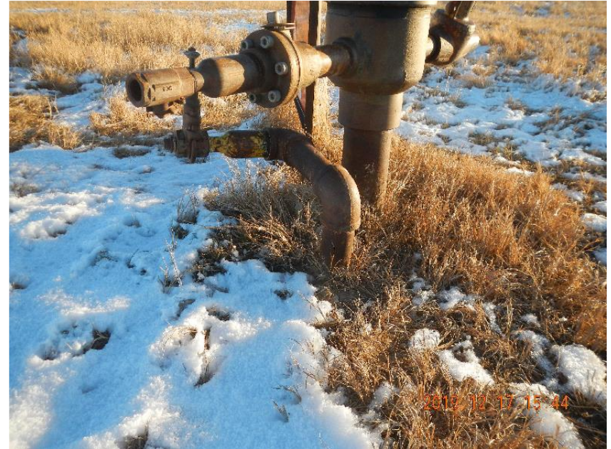
Photo 4: View of additional riser.
