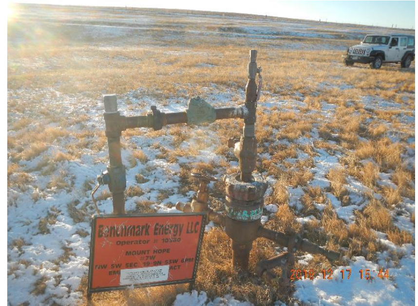
Photo 2: Wellhead and tree.
