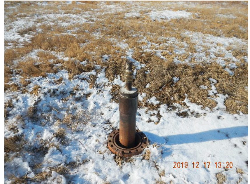
Photo 2: Wellhead with no tree. Surface casing is open to atmosphere.
