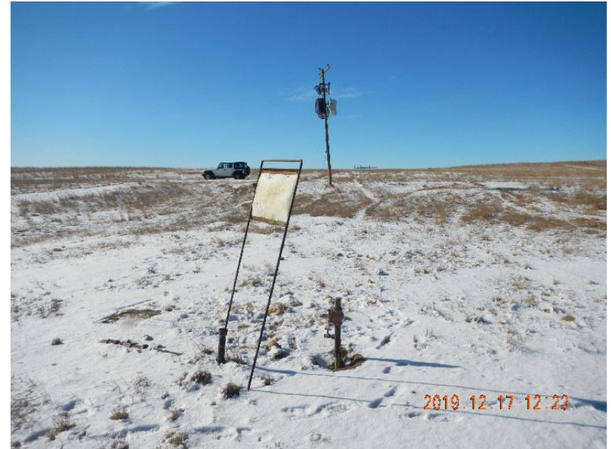
Photo 4: View from wellhead looking towards power pole with transformers.
