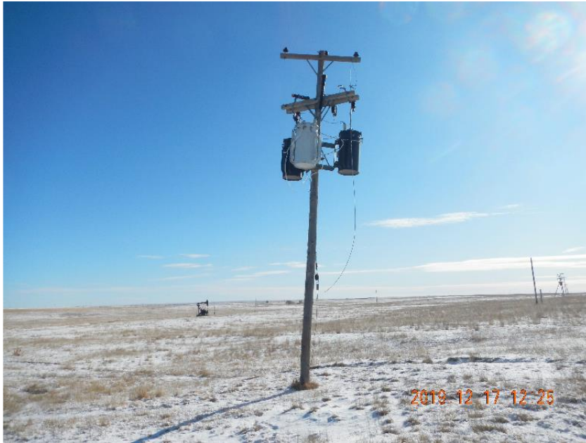
Photo 5: Power pole with transformers.
