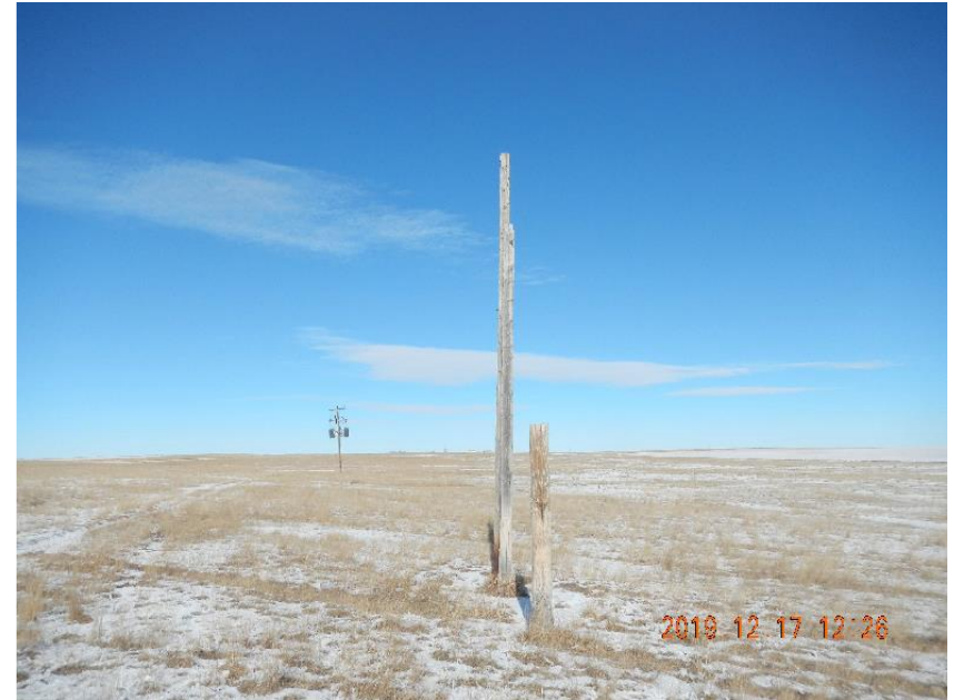
Photo 6: Power poles at location.
