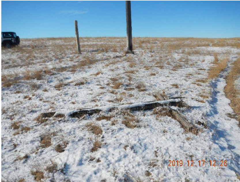
Photo 7: Broken off power pole top on ground.
