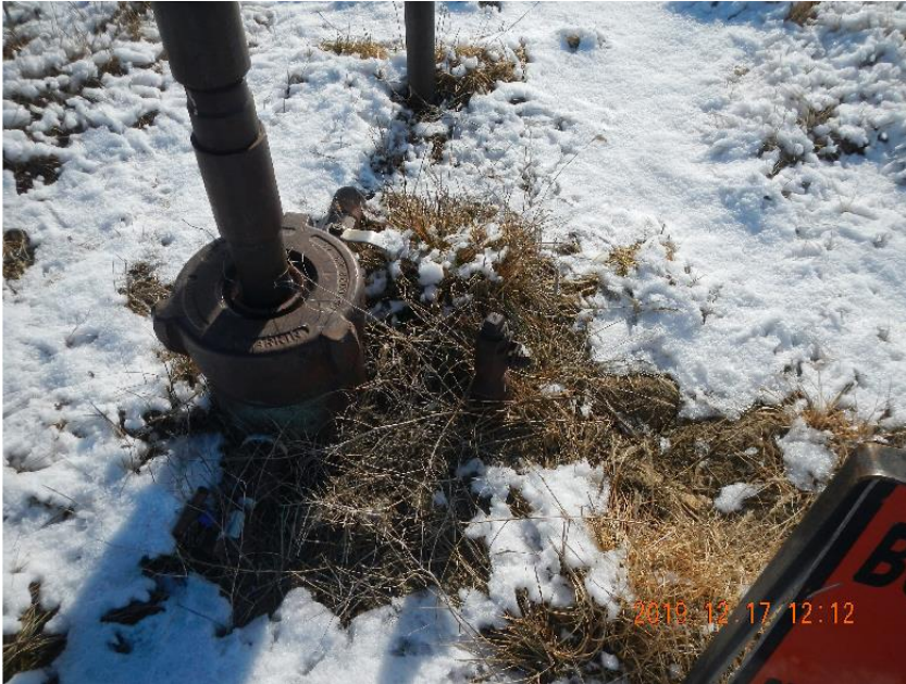
Photo 3: Additional view of wellhead and risers.
