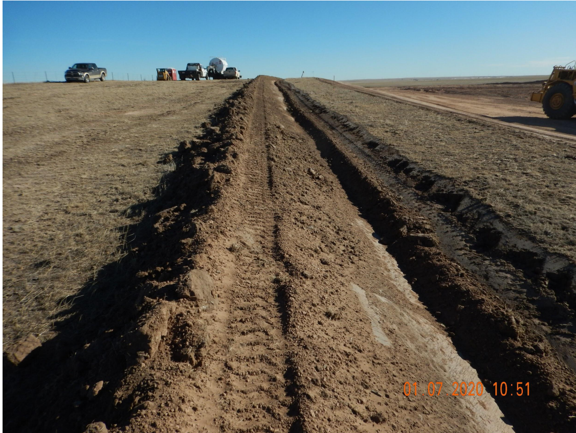
Photo 6. Photo taken from the northwestern perimeter of location, facing East. Photo illustrates a ditch and berm BMP. Berm portion of the BMP has not been installed in accordance with good engineering practices, as the berm has been left unconsolidated.
