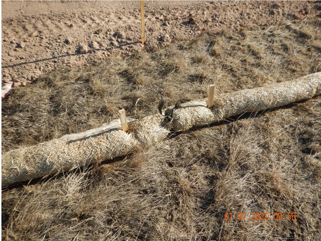
Photo 2. Photo taken from the entrance of location. Photo illustrates the wattle BMP has not been properly installed. Wattle BMP shall be trenched and back-filled and the ends shall overlap.
