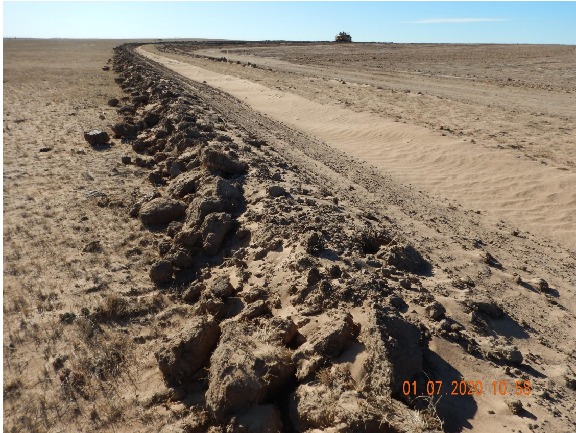
Photo 10. Photo taken from the eastern perimeter of location, facing South. Photo illustrates soil particle deposition accumulation within the ditch BMP and the unconsolidated berm BMP.
