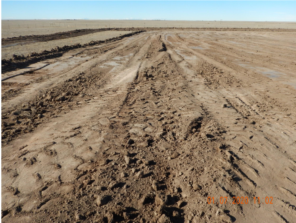
Photo 12. Close up photo taken from the southern location, facing West. Photo illustrates Operator is in process of conducting topsoil salvage operations. Based on field observations, it appears the Operator is salvaging to the appropriate depth.
