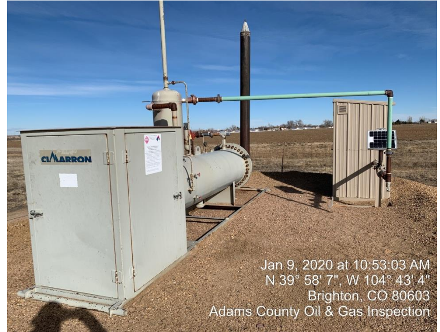
Photo# 2 Separator and Meter house
