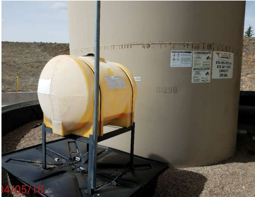
Previous inspection signage missing
