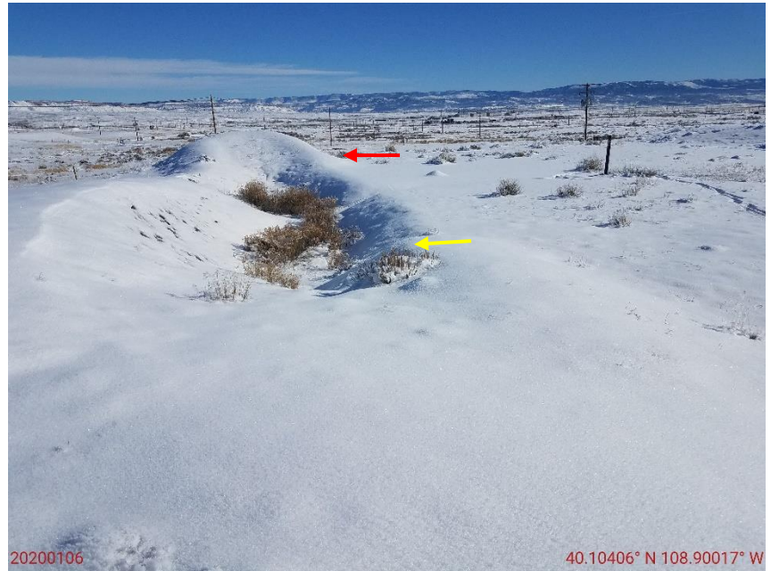
Photo 4: Photo taken from the south end of the location, facing east. Photo shows an open pit on the north end of the location (yellow arrow), and the excavated soils (red arrow).
