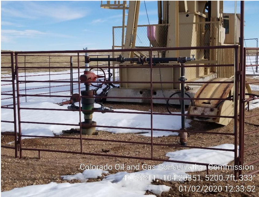
Photo 1 – Wellhead and Pumping Unit
