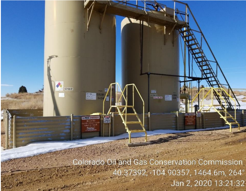
Photo 5: Centralized Tank Battery
