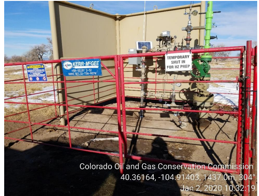
Photo 2: Wellhead; equipment connected
