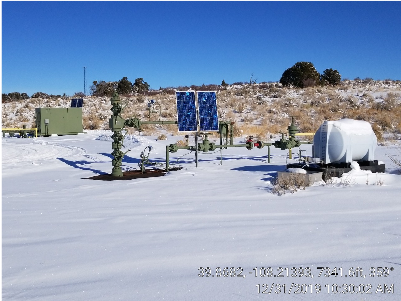
Photo 2. Well head & separator.
