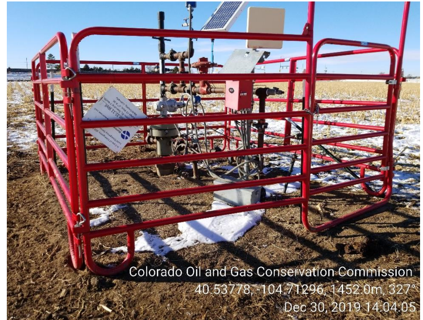
Photo 2: Wellhead ; WEEDS REMOVED
