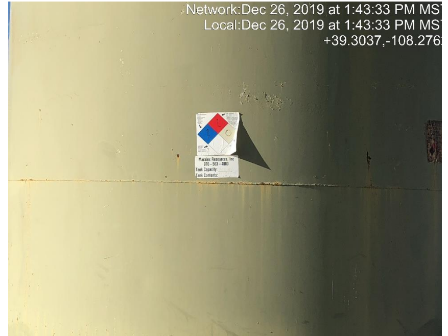
Photo #0308 Tank capacity and contents not legible.
