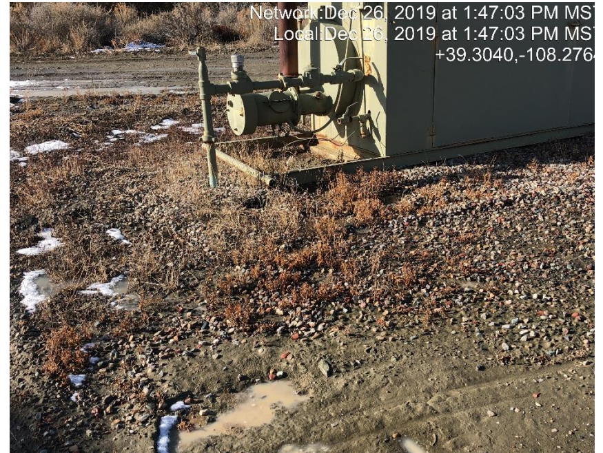
Photo #0310 multiple place with weeds on location.
