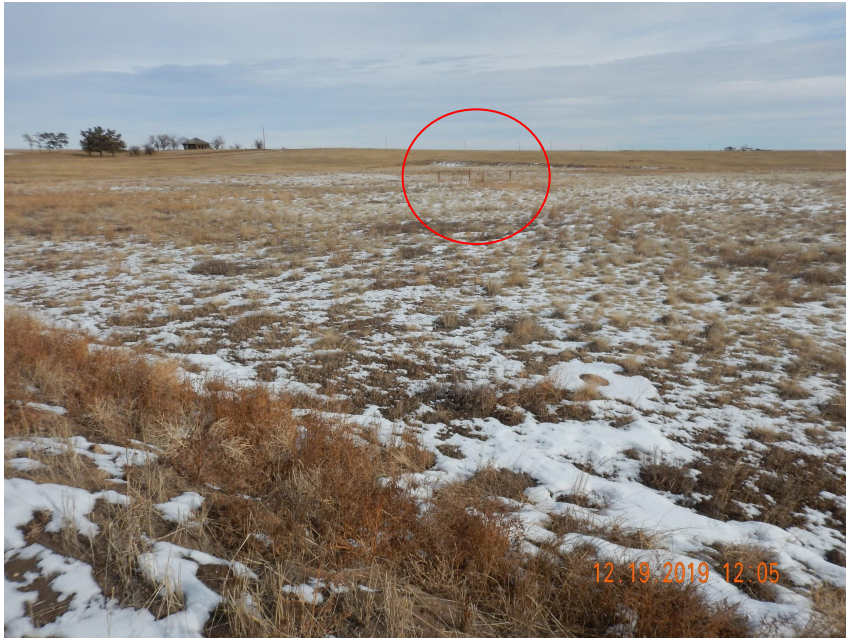
Photo 3. Photo taken from the western well pad, facing Northeast. Photo illustrates Operator has failed to plug and perform Final Reclamation.
