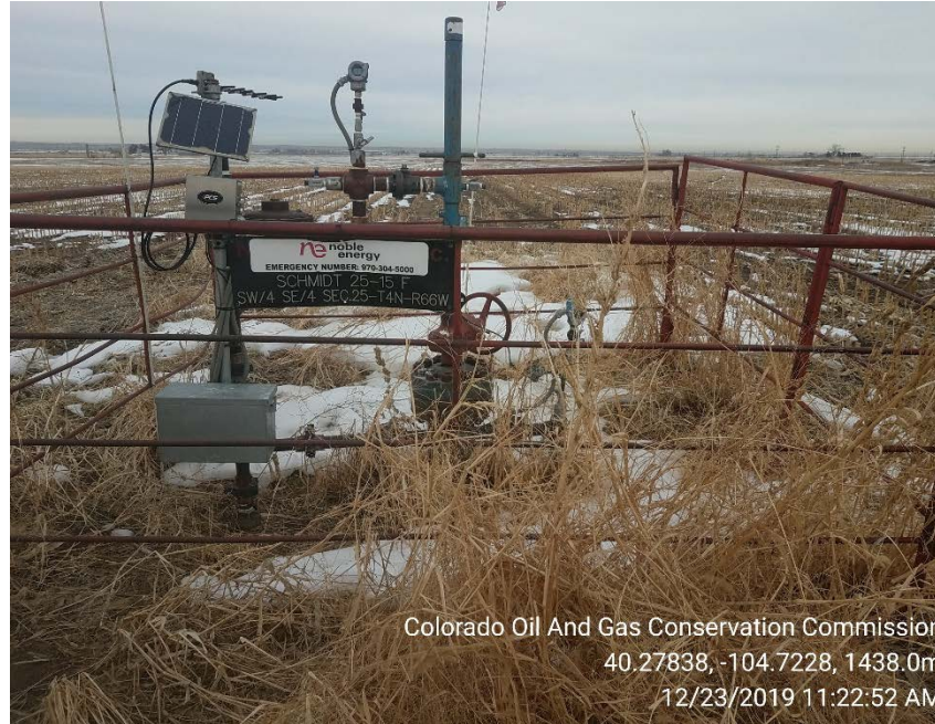
Wellhead and debris
