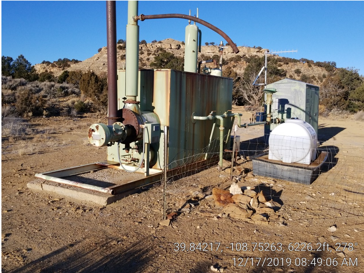
Photo 2. Separator & meter building.
