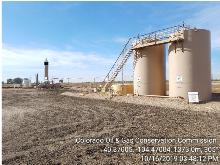
Photo #3 Rothe 43-30, 44-30 Battery Shut-down | Inactive prior insp.
