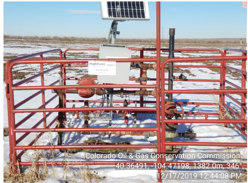
Photo #2 Rothe 44-30 Wellsite Temporarily Abandoned | TA Sign with well name NOW posted
