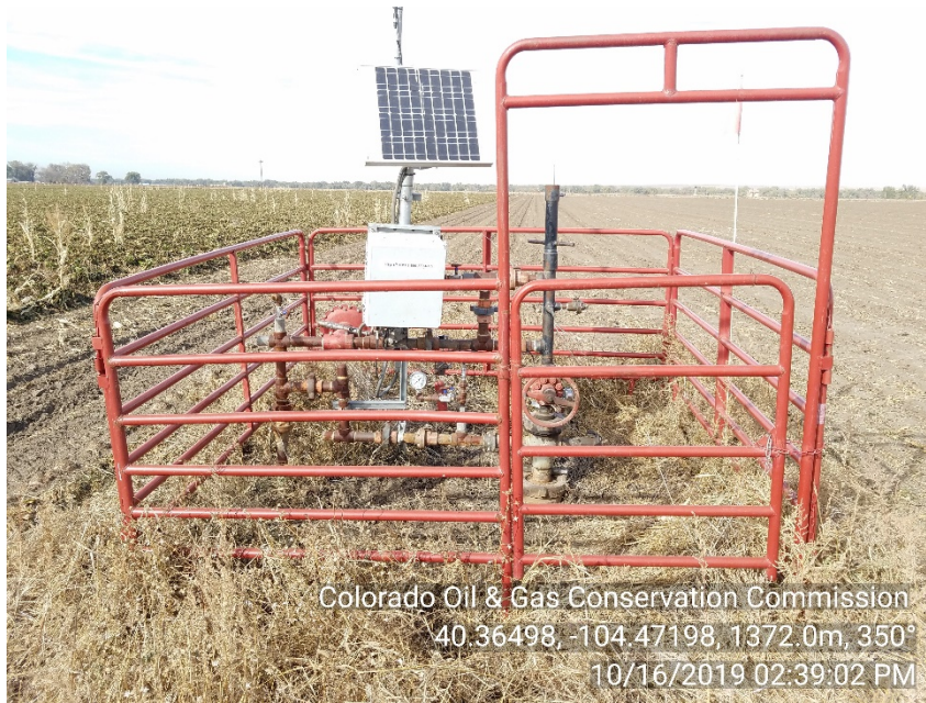
Photo #1 Rothe 44-30 (05-123-32101) Wellsite Temporarily Abandoned | TA Sign with well name NOT posted prior insp.
