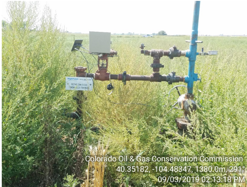
Photo #1 Rothe CSW-31 (05-123-23945) Wellsite Temporarily Abandoned | TA Weeds prior insp.
