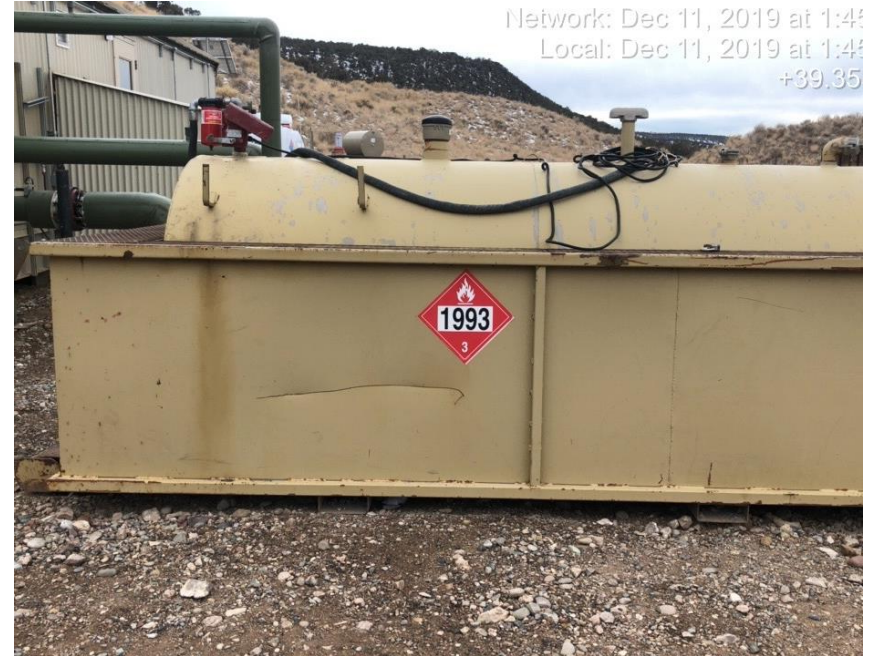
Photo #0229 Diesel tank capacity not labeled.
