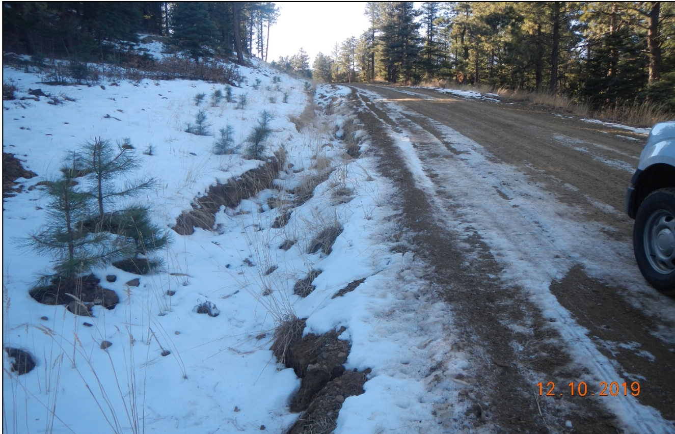
Photo 1. There is signs of erosion occurring along the road at Lat/Long:37.209713, - 104.935704.
