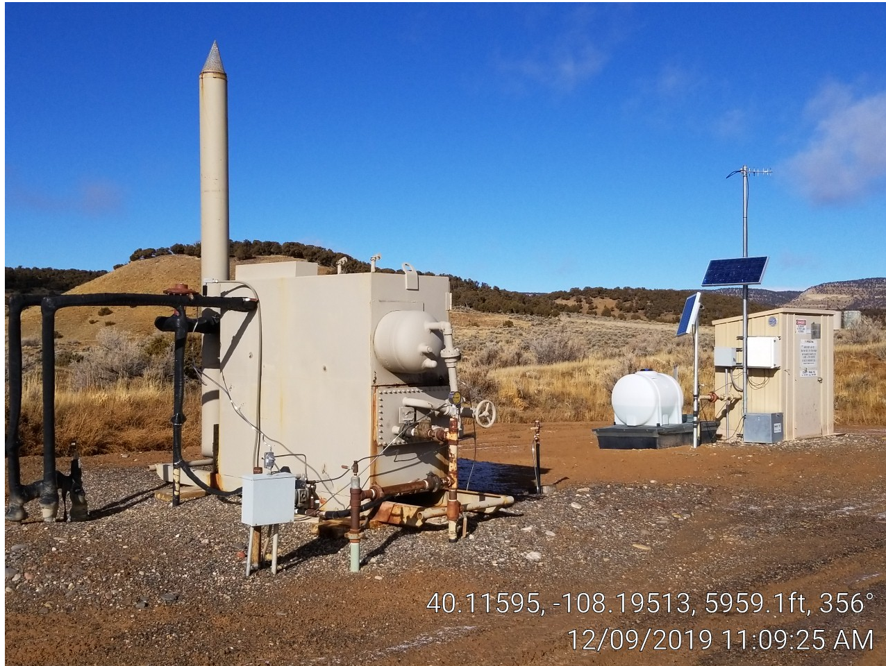
Photo 3. Separator & meter building.
