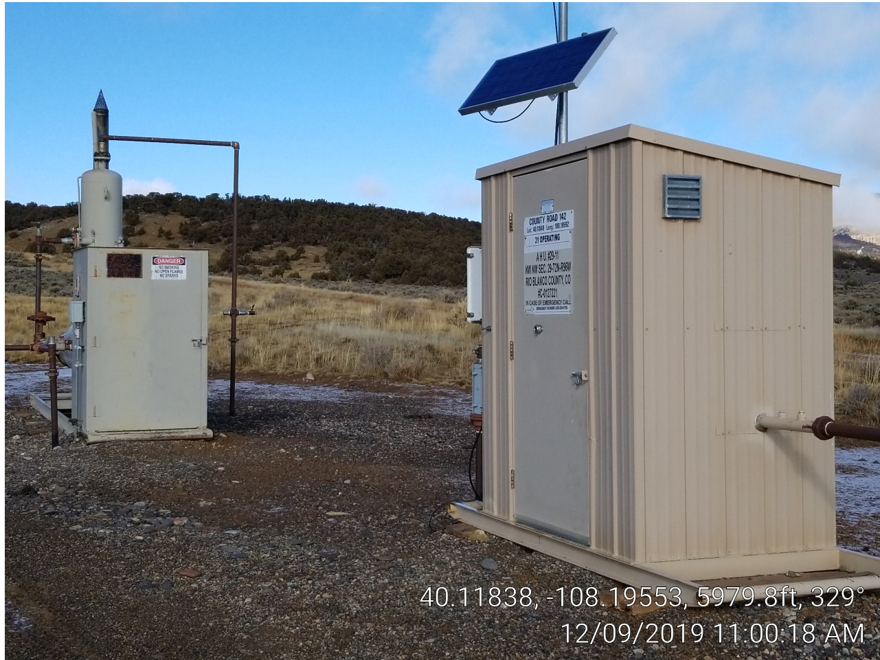
Photo 3. Separator & gas meter building.
