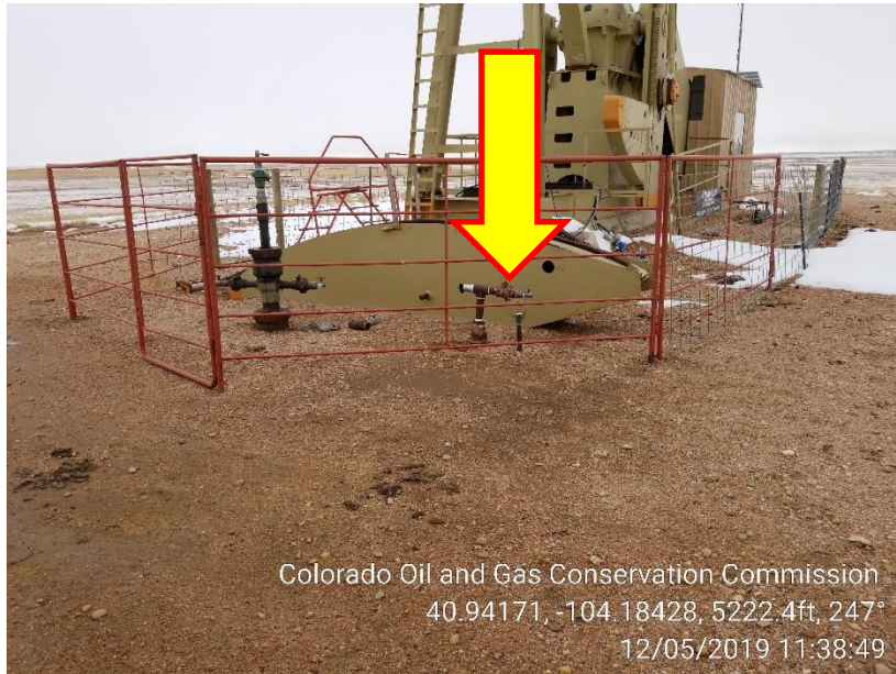
Photo 3 – Unmarked 2” and 1” Risers
