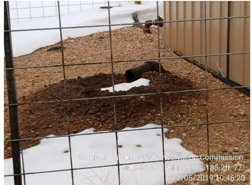
Photo 2 – Stained Soil at Exhaust
