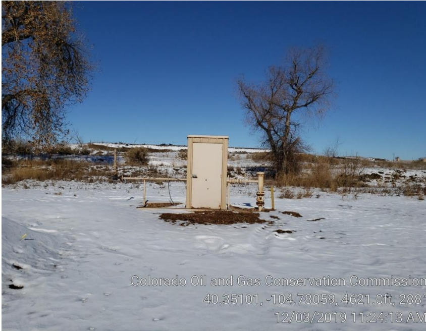
Photo #2 Gas Meter Run
