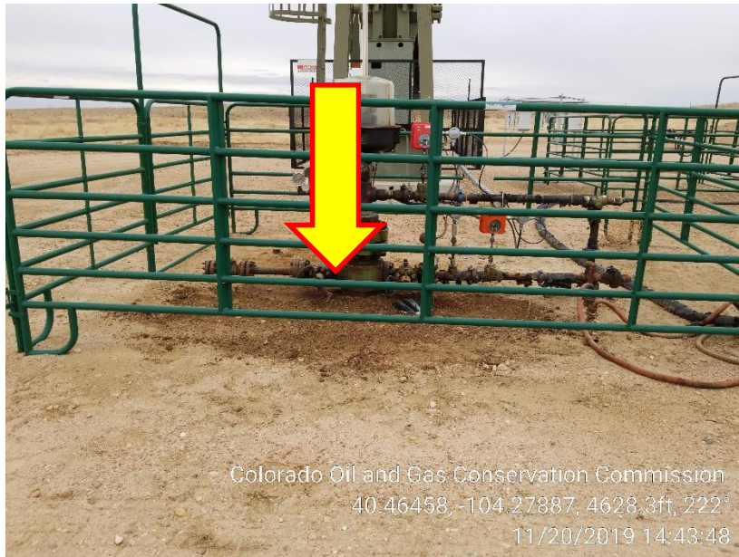
Photo 3 – Stained Soil at Wellhead
