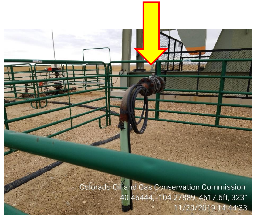
Photo 4 – Unmarked 3" Riser at Pumping Unit
